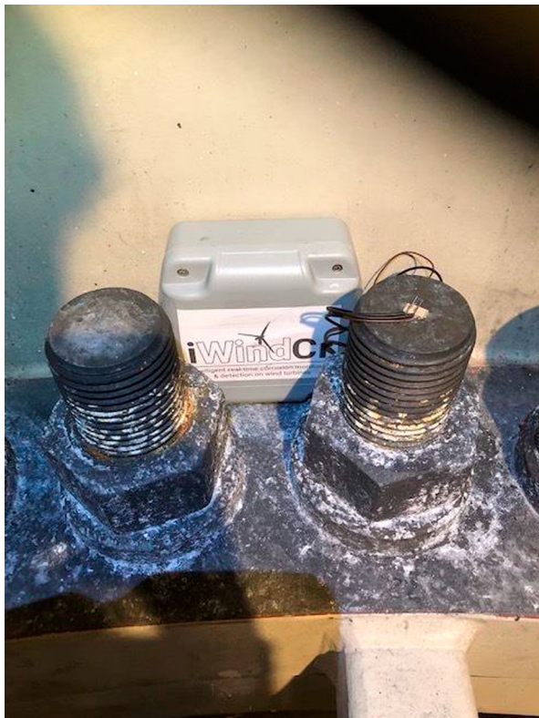
Figure 2. iWindCr system set-up in the MP-TP flanged connection location with the sensor attached to the M72 stud on the right.
