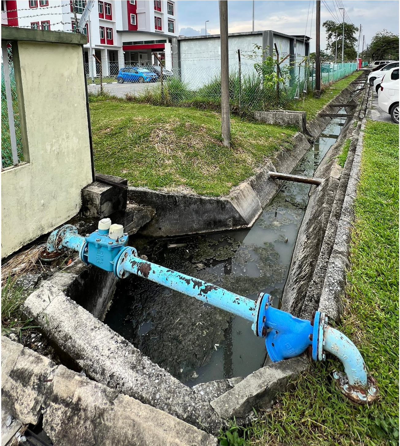
Figure 1. Improper drainage blockage issue in a commercial area, highlighting the presence of potential unwanted pollutants if not properly treated
