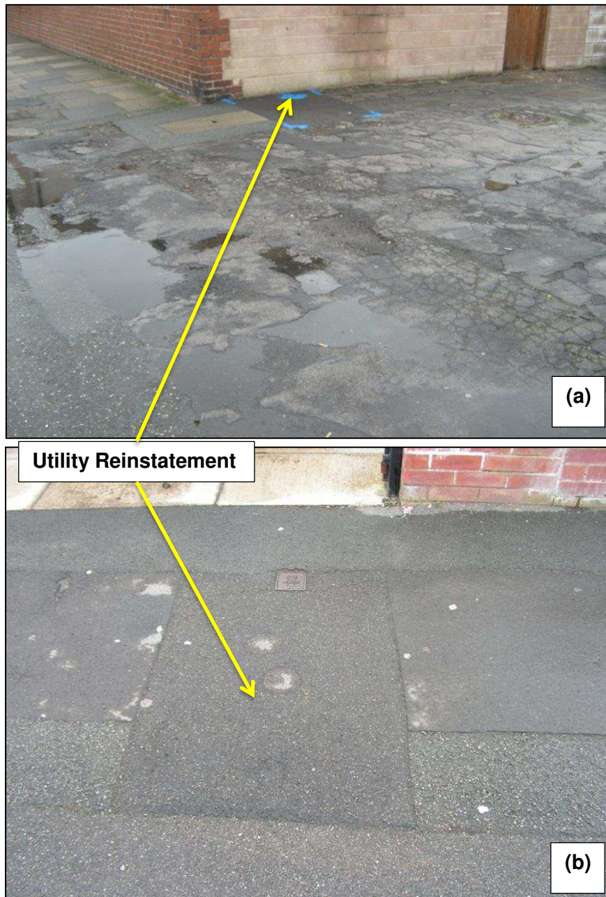
Figure 6: Satisfactory performance of reinstatements works even comprising SROH non-compliant air voids contents. Photograph taken; (a) after 27 months of installation, (b) after 12 years of installation [43]
