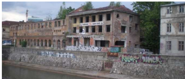
Figure 5. Buildings that were burnt out and never restored along the Miljacka River (photo by lead author)
