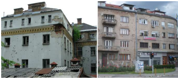
Figure 3. Bullet holes and the scars of war noticeable in the façades of buildings (photos by lead author)
