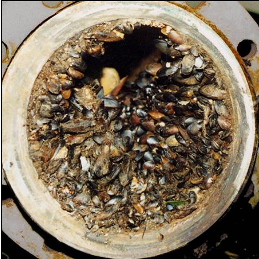
Figure 7.4.1. Biofouling at a Flange of a Sea Water Pipe 40
