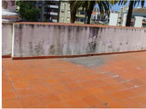
Figure 6 - Terrace covering with ceramic roof tiles. Water accumulation due to insufficient slope of the terrace floor.
