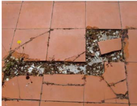
Figure 7 - The inexistence of expansion joints at the ceramic tiled floor leads to its fracture and to the cracking of cement based mortar layer under tiles, contributing for inefficient roof water proof and therefore leading to leaching of the mortar joints between brick masonry vault.
