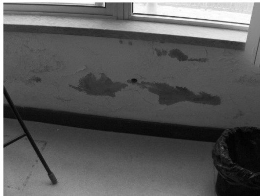
Fig.5: Example of the condensation effects at the first floor of the building school.
