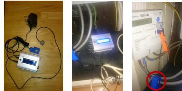
(a) Energy monitor configured to smart meter sensing specifications (b) Energy monitor installed in a patient's home (c) Current transformer clip (red circle) fastened around the live cable
