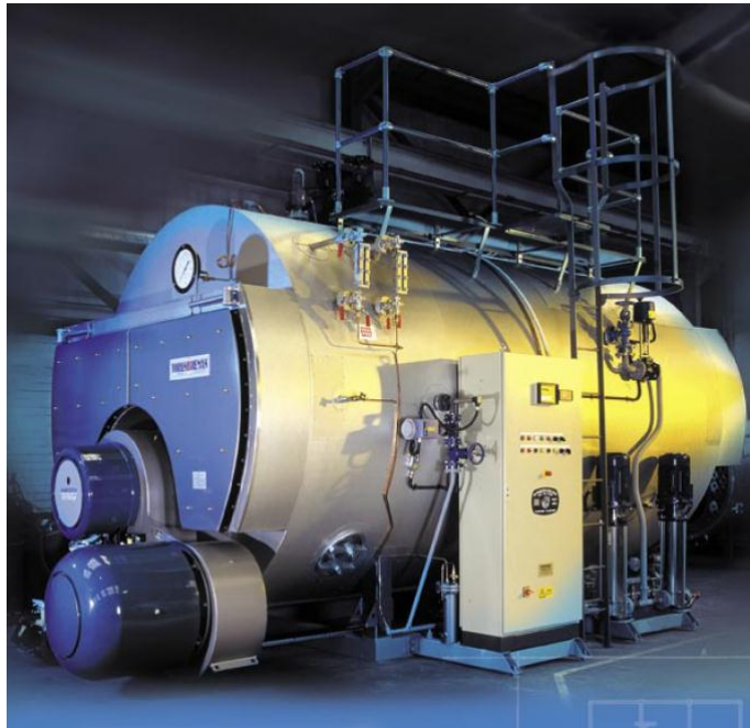
Fig. 4 Byworth steam boiler – University of Manchester Wythenshawe Hospital
