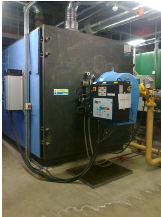
Fig 2. MTHW boiler – The Royal Derby Hospital
