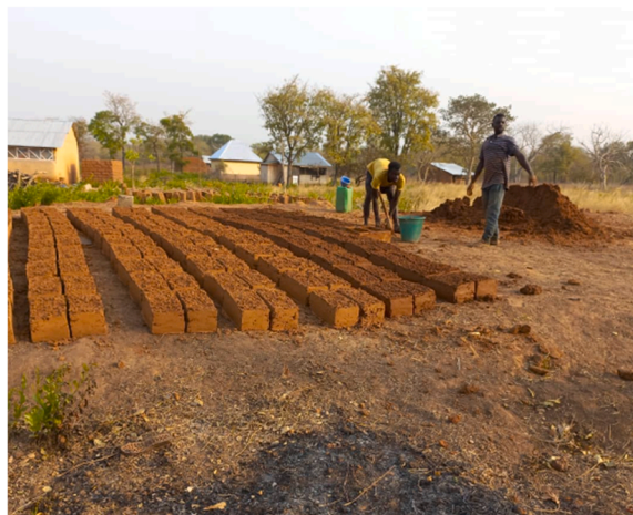
Fig. 2. Reddish Clayish soil used for plaster and blocks preparation in Wa, 2022 (photograph by the authors).
