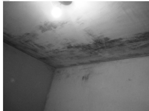
Figure 14: Example of the condensation effects at the first floor of the dwelling.
