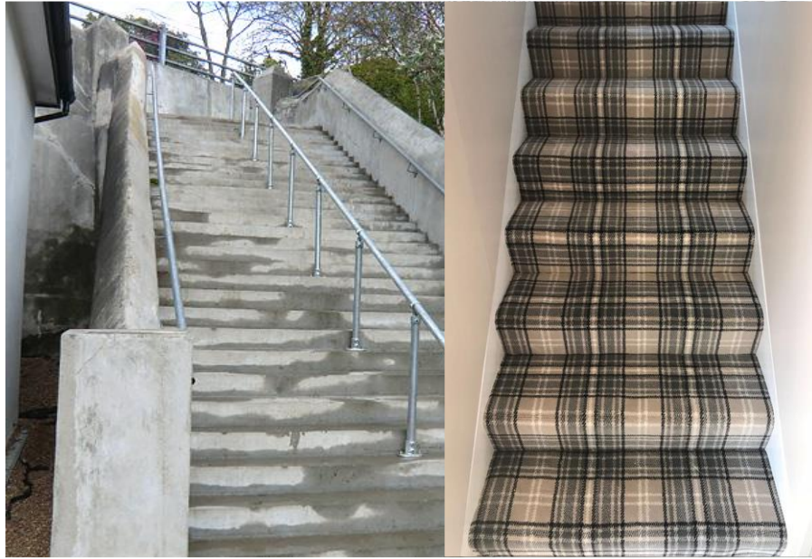
Figure 1.2 Examples of stairs uniform in appearance or covered in patterns that make it difficult to discern the step edge.
