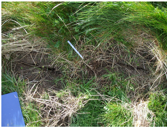
Figure 5. Photograph of crack #10, a representative embankment crack.
