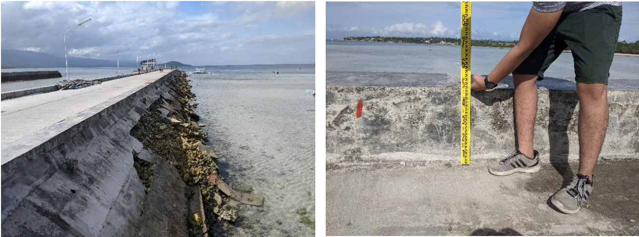
Figure 8. Left. Damage to port pier at Moalboal. Right. The storm surge level reached the top parapet on the side of the port pier.
