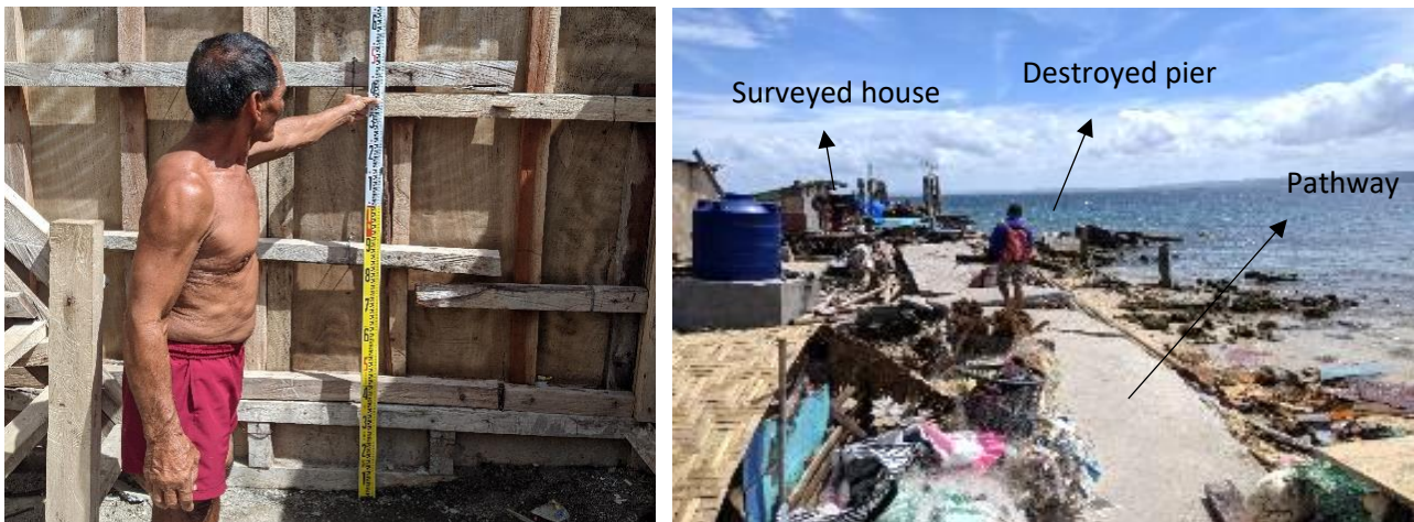
Figure 11. Left. A resident indicates the level of the water in front of the barangay hall. Right. At the right side of the photo is one of the houses surveyed in front of what is left of the pier (structure on the right side)
