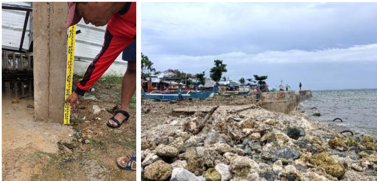
Figure 15. Left. Inundation level in front of the basketball court of barangay Santo Rosario. Right. New (far side of picture) and old (close side of picture) seawall at barangay Tugas.
