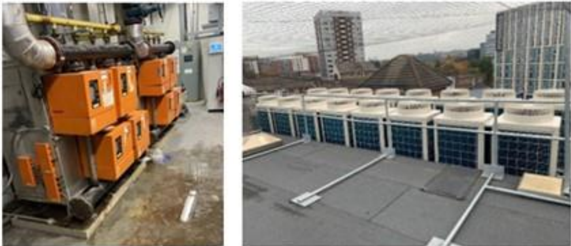
Figure 3 Space requirements for boilers and air source heat pumps Henry Cotton
