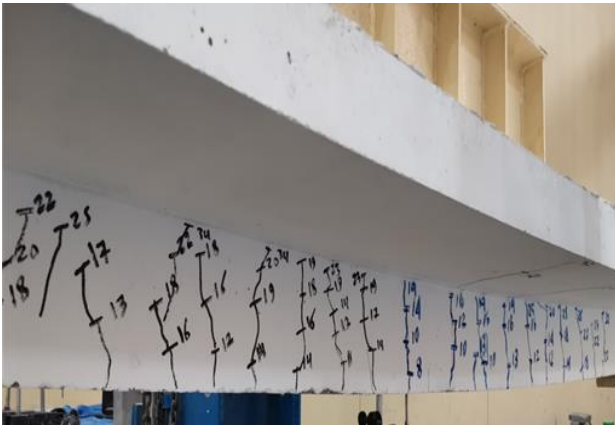
Fig. 13. Crack pattern of OWRS3
