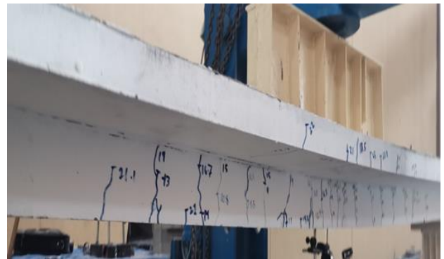
Fig. 12. Crack pattern of OWRS2
