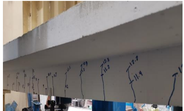
Fig. 11. Crack pattern of OWRS1
