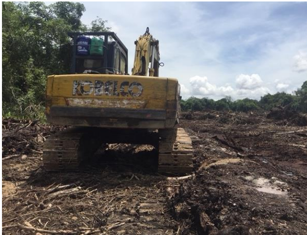
Figure 1 The use of excavator for land clearing and the preparation of oil palm plantation site in Sibul, Sarawak, Malaysia
