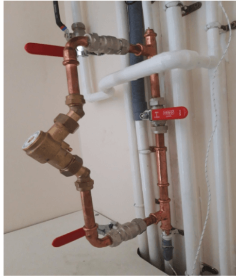
Figure 3. CombiSave valve in use and temperature sensors.
