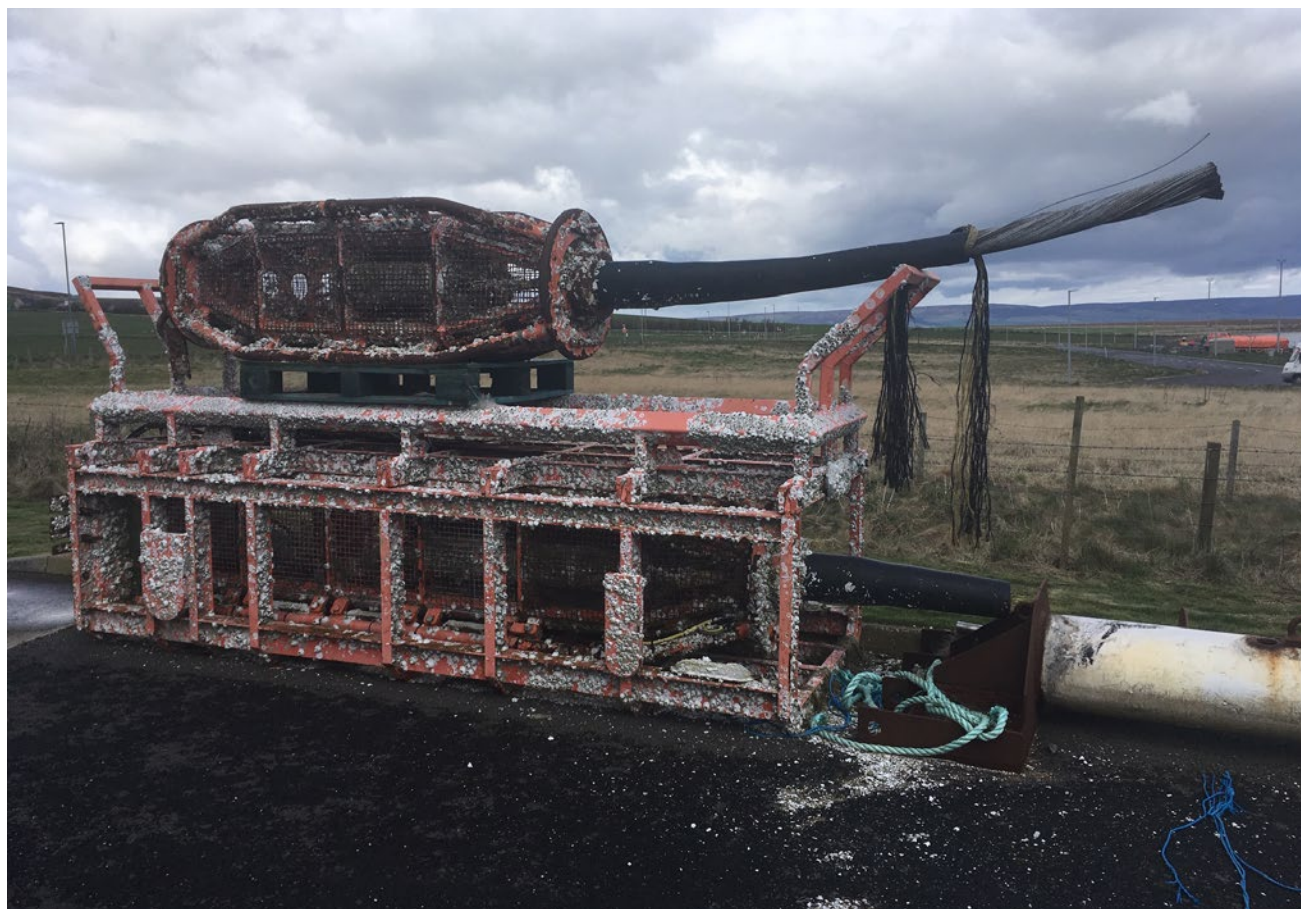
Figure 15. Two electrical connection hubs, one on top of the other, used at the wave test site of EMEC (Orkney, Scotland) and expanded view of barnacle colonization after three years at sea.
