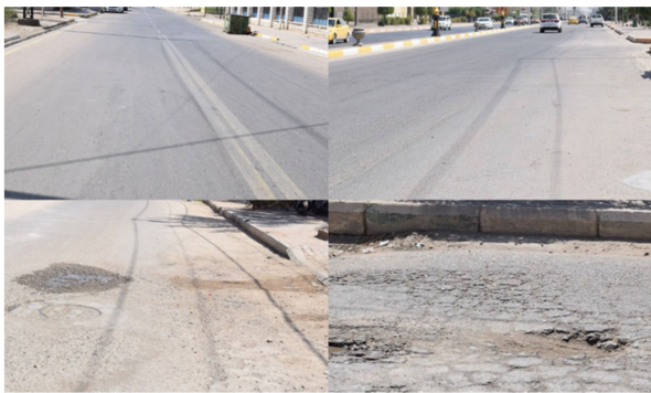
Figure 4. Common pavement conditions of the study area, a) very good, b) good, c) fair, d) poor.
