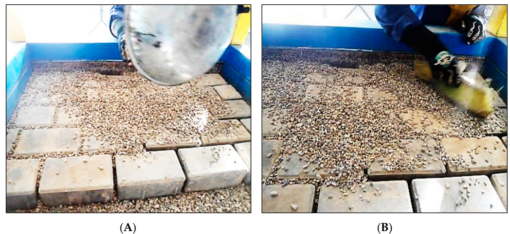
Figure 19. Finalizing process of PICP surface pavers. (A) Filling process of joints [27]; (B) Sweeping and distribution [27].
