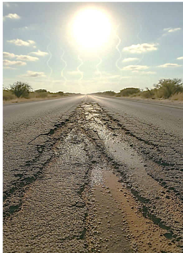
Figure 1. Heat-induced distress on asphalt pavement in hot climate regions.
