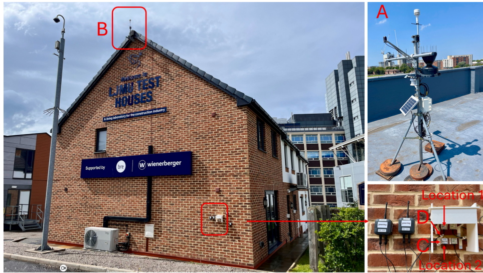
Fig. 3. Outdoor nodes mounted on the building east façade. A. HOBO RX3000 weather station Advanced Kit with BF5 diffuse radiation sensor (71 meters away from the site, on the roof of nearby building). B. HOBOnet Wireless Ultrasonic Wind Speed & Direction Sensor for local wind measurement. C. greenTEG outer surface temperature sensor. D. greenTEG outer air temperature sensor.
