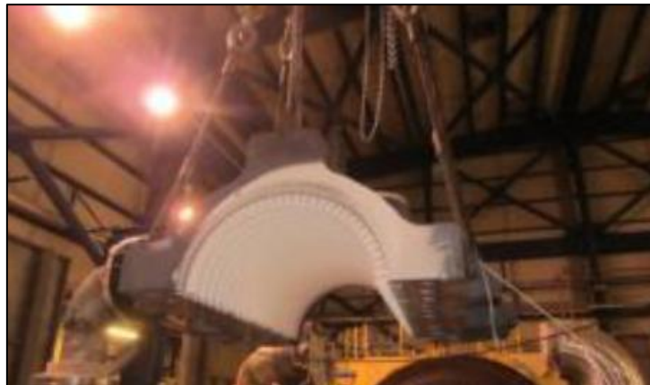
Figure 8. High-pressure steam turbine casing
