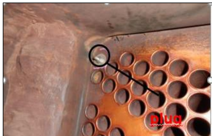
Figure 9. Detached plug found in the condenser waterbox
